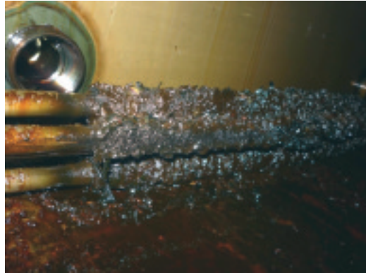
Figure 2 Significant deposits on a heating element due to extreme temperatures
